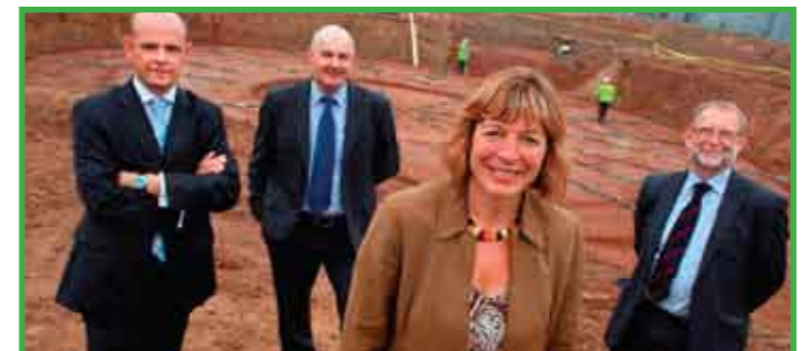
Work begins on the £5m anaerobic digestion plant at the RF Brookes' ready meals factory
