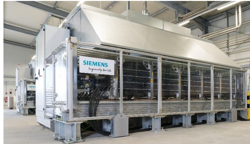
Image: Siemens, PEM electrolyser, Germany, 2015
